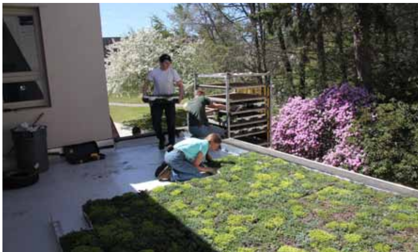
Green Roof being installed at the Crozier Williams College Center by Arboretum Horticulturist Leigh Knuttle (kneeling) and Brendan Kempf '10 (standing). The project was designed by Brendan and funded by the Sun Hill Foundation.
